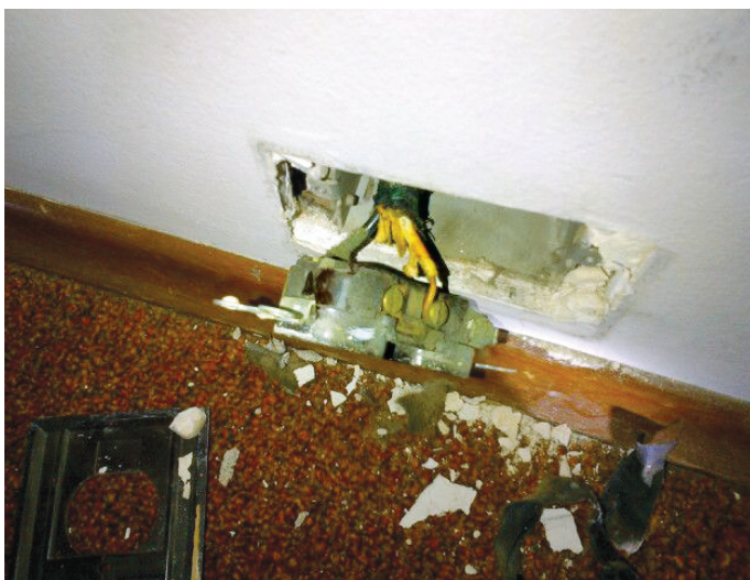
3-prong outlet on ungrounded cable
