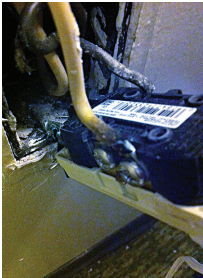
Aluminum wire on copper outlet
